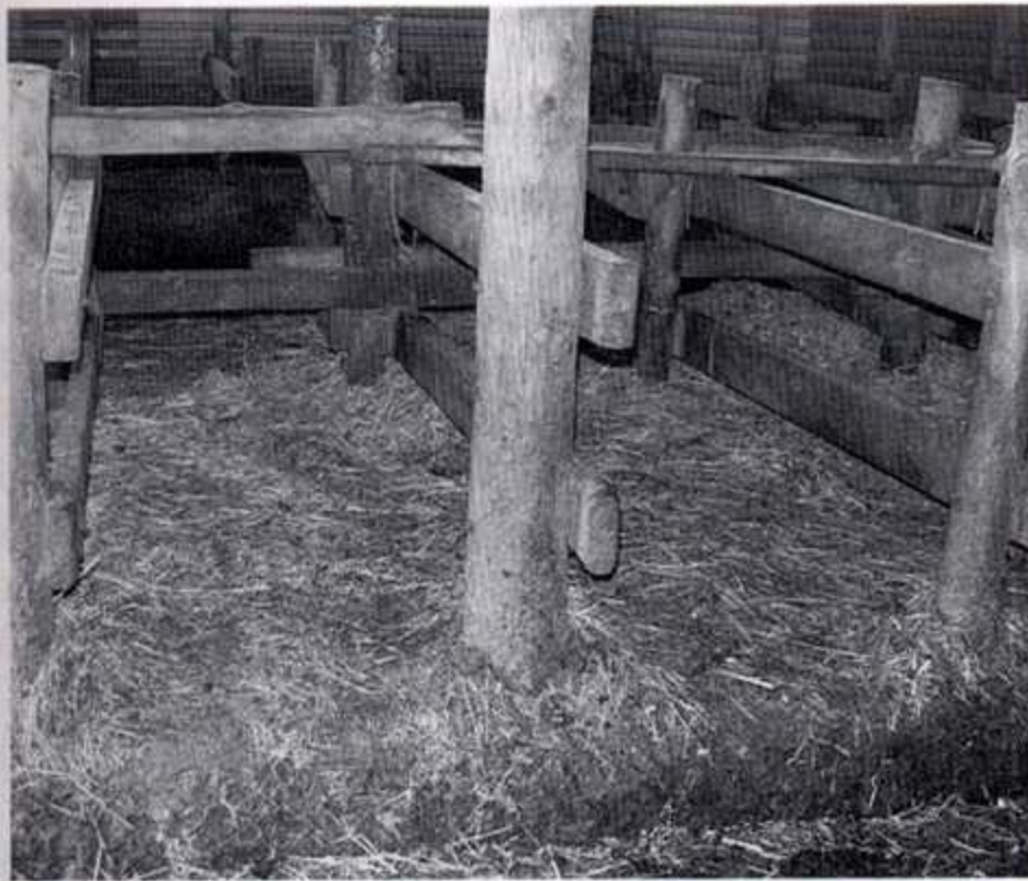
FIGURE 6.8 Excessively narrow home-made cubicles. The cows found these uncomfortable.
